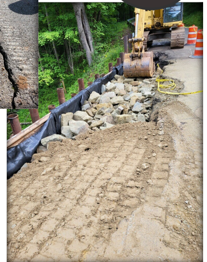
Slip on County Road 17 due to heavy rains during the April 2024 flooding
